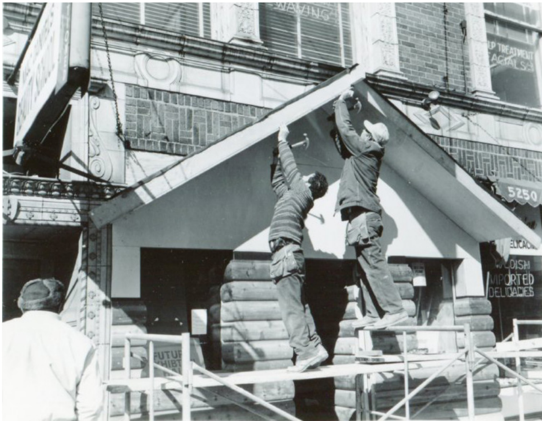
Construction work on the original Museum log cabin façade at 5248 North Clark Street
